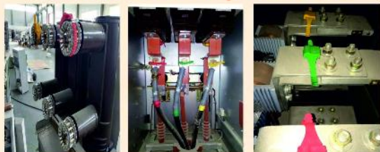
Wireless Sensor strapped to Bus bar
